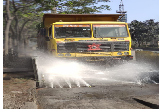
Wheel washing System
